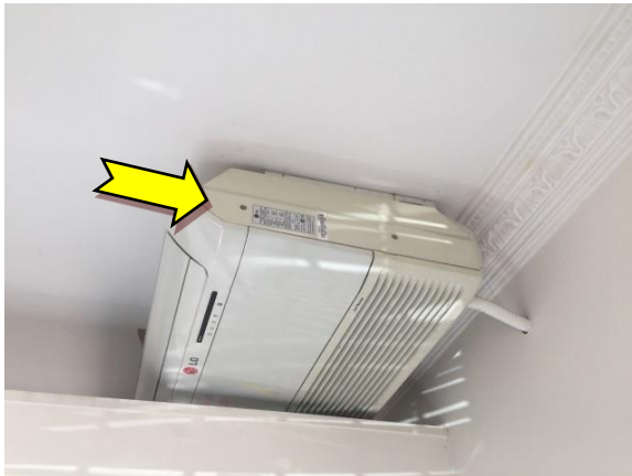
Photo 3. Interior, ground level, office, air conditioning unit – R22 ODS-containing refrigerant.
