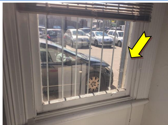
Photo 6. Interior, ground level, throughout, window frames – lead-containing white upper paint systems.
