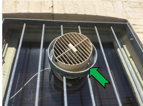
Photo 2. Exterior, ground level, east elevation, north window, window mounted extractor fan – non asbestos-containing mastic sealant.
